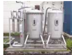
Groundwater purification system, Tokyo Hachioji Site
