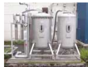
Groundwater purification system, Tokyo Hachioji Site
