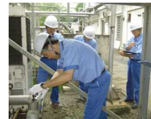
Risk assessment for non-routine work
