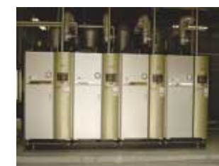
Natural gas boilers
